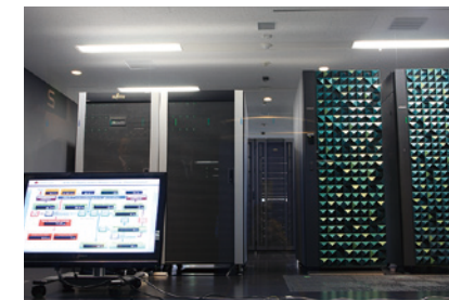
▲ Multicore servers installed in the server room
