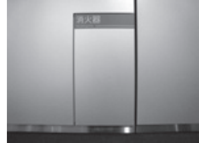
Figure 1-4-1. Example of a place where a fire extinguisher has been installed
