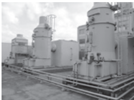
Figure 3-3-6. Scrubber facilities on the rooftop
