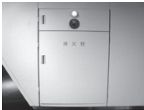
Figure 1-4-2. Example of a place where an indoor fire hydrant has been installed
