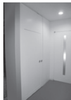
Figure 1-4-4. Fire doors (large and small) which close when the fire alarm goes off
