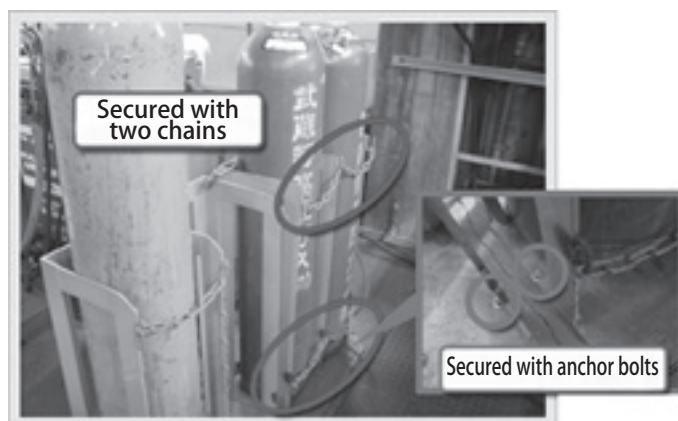
Figure 3-4-5. Securing high-pressure gas cylinders
