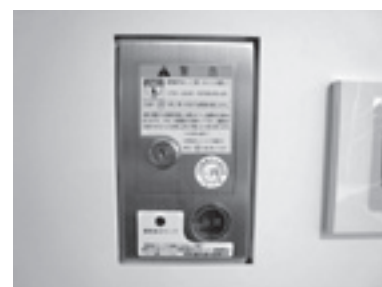
Figure 1-4-7. The fire shutter operating panel
