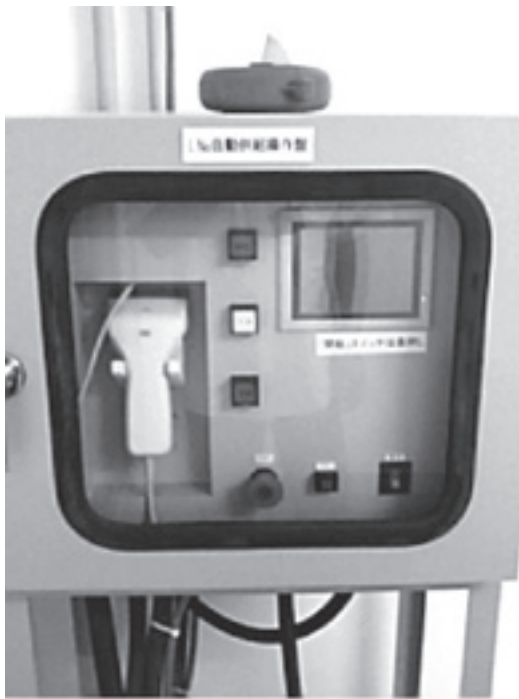
Automatic dispenser control panel
