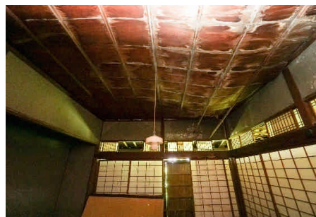
fig.2 林邸1階天井現状
